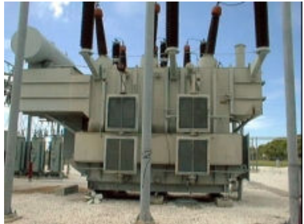
Figure 3. Image of an high voltage transformer
